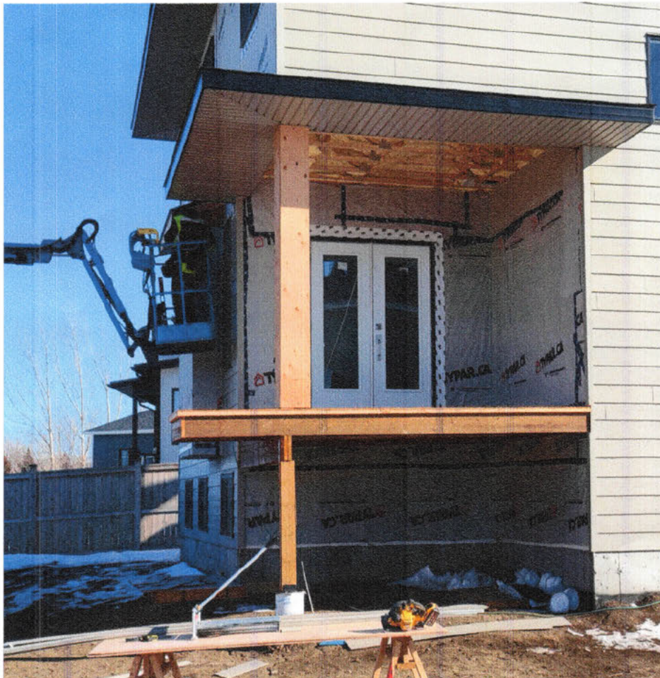
The house is fully completed now with steps going down the side of the house This picture was from during construction
